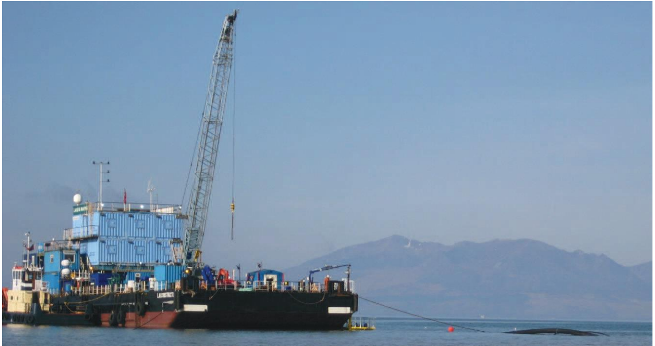
Figure 31. Large barge with four point anchoring. On the right hand side of the barge the duct can be seen being pulled into the HDD. The water depth is approximately 4m.
